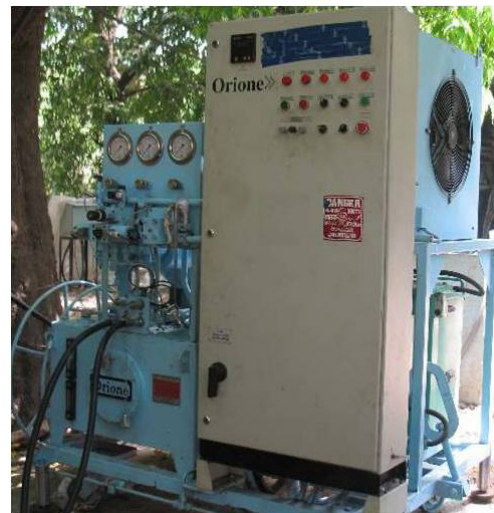
Fig. 8: 30 kW oil hydraulic power pack.
