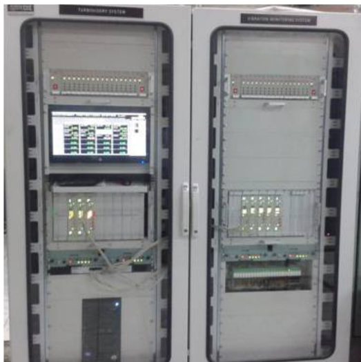
Fig. 5: MPS systems installed at NTPC, Kahalgaon.
