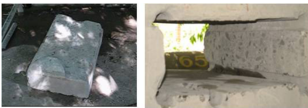
Fig. 13: Concrete block removed from the wall & opening after removal of the block
